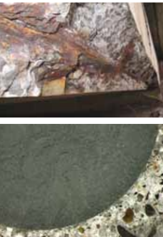
◀ After a comparable service life, the corrosion of the oxidized steel rebar has degraded the concrete around it, while the V•ROD rebar is intact and surrounded by healthy concrete.
